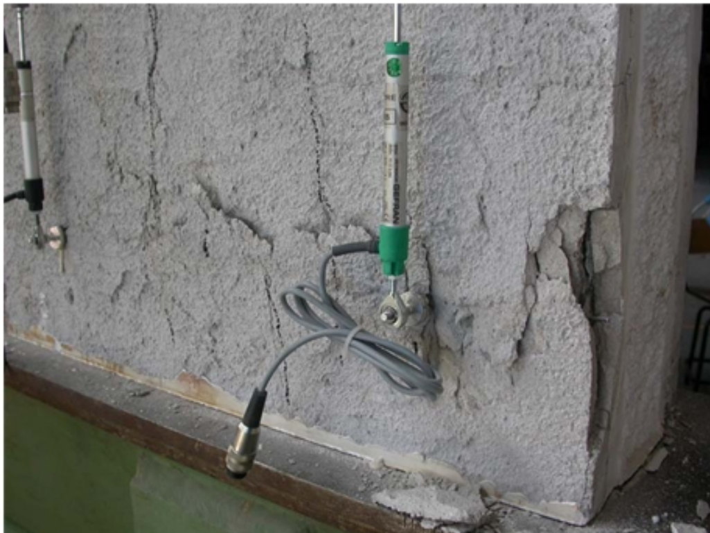
Figure 15: Breakage due to cement compression
