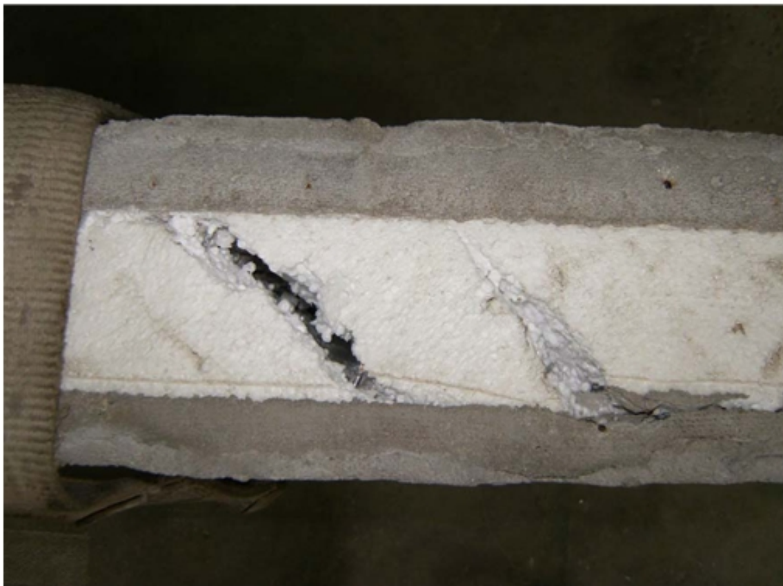
Figure 24: Diagonal fissures in the polystyrene
